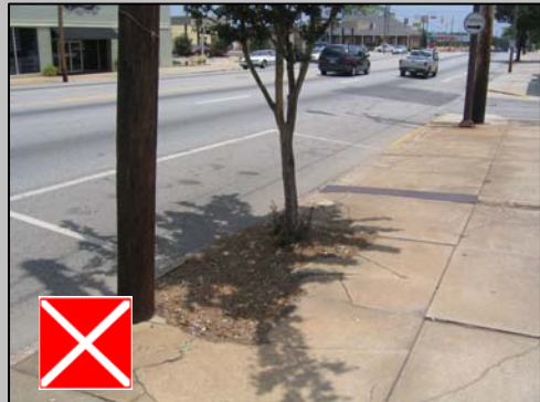
Neglected tree maintenance
